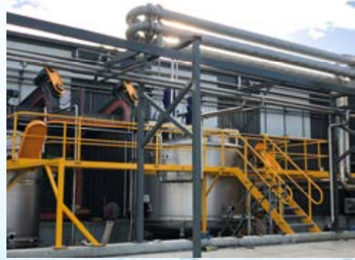
Mixing Tank 3&4, Established 2018
