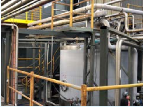
Mixing Tank 1, Established 2006
